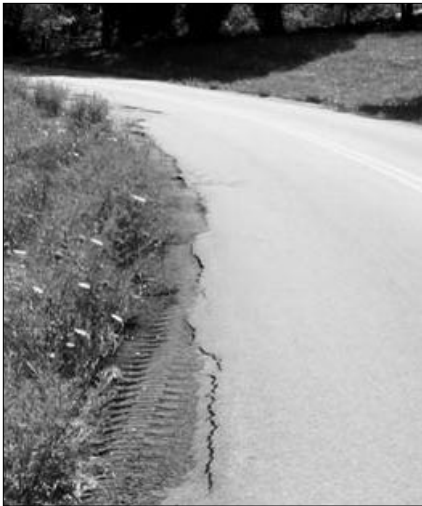
This shows a classic shallow fill failure. If the fill has some strength, launched soil nails will fix the problem.
