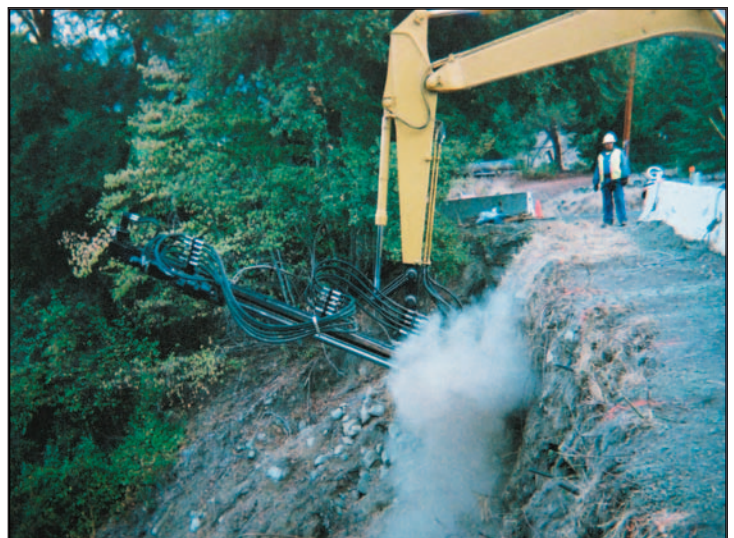
Below: Soil Nail Launcher in action at the Hawkins Bar Road slide in Trinity County, Northern California
