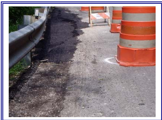
Stocking Road Slip – Developed an 18" vertical failure in the pavement.
